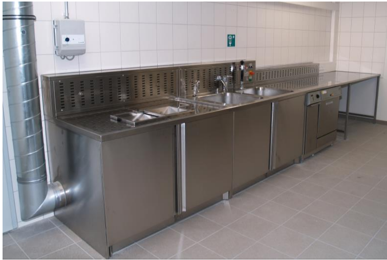
Individual solution with basin, disinfection system and working table
